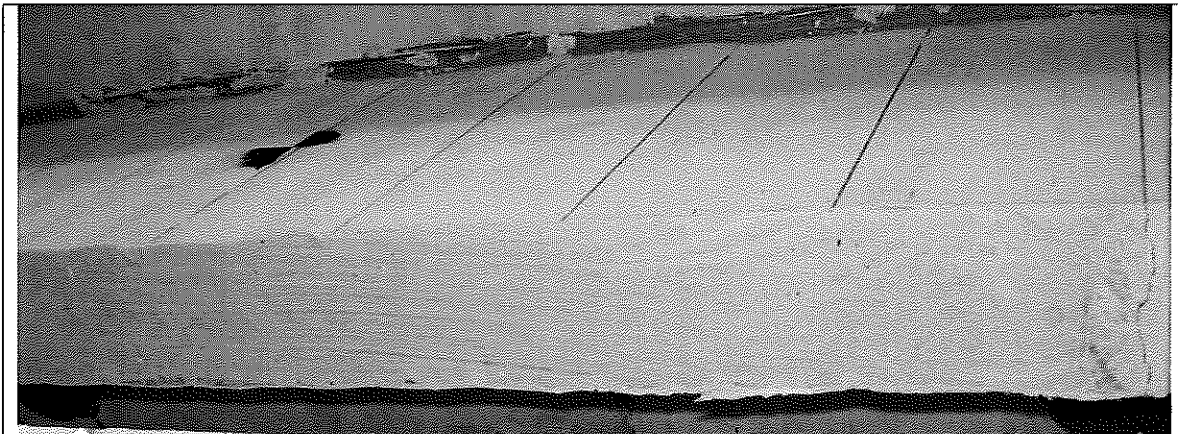
Figure 10— Hairline flexural crack at the right corner of the beam after VERTEQII-250%
