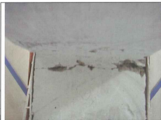
Figure 9a — Crack at the upper right corner of the opening after VERTEQII-225%
