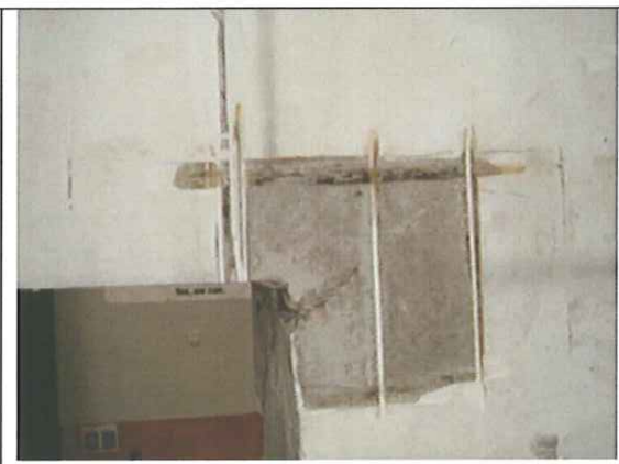
Figure 9b — Part of OCFS taken off, diagonal crack found after VERTEQII-225%
